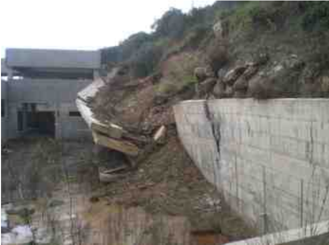
Fig. 6 - Collapse of the retaining walls
