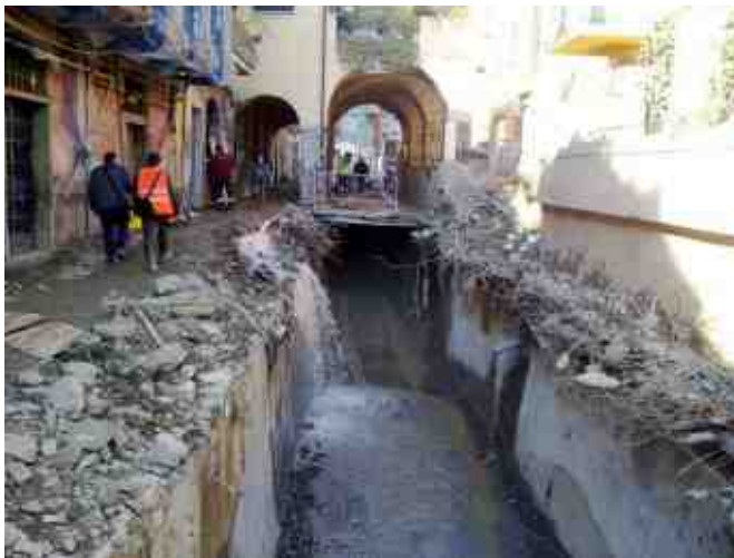
Fig.1 – Underground waterway “exploded” during the flood event occurred in November 2001 (Monterosso al Mare - SP).
